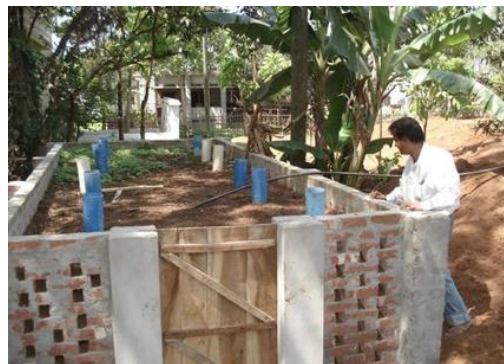
Fig. 2. Brick-built tank constructed for disposal and decomposition of coir pith into organic fertilizer
